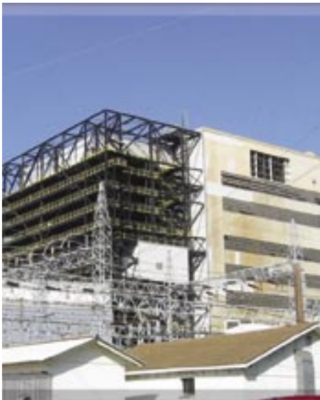
Plant Gorgas, Alabama Power Company Unit 10 has an SCR that has been operating for three ozone seasons.
