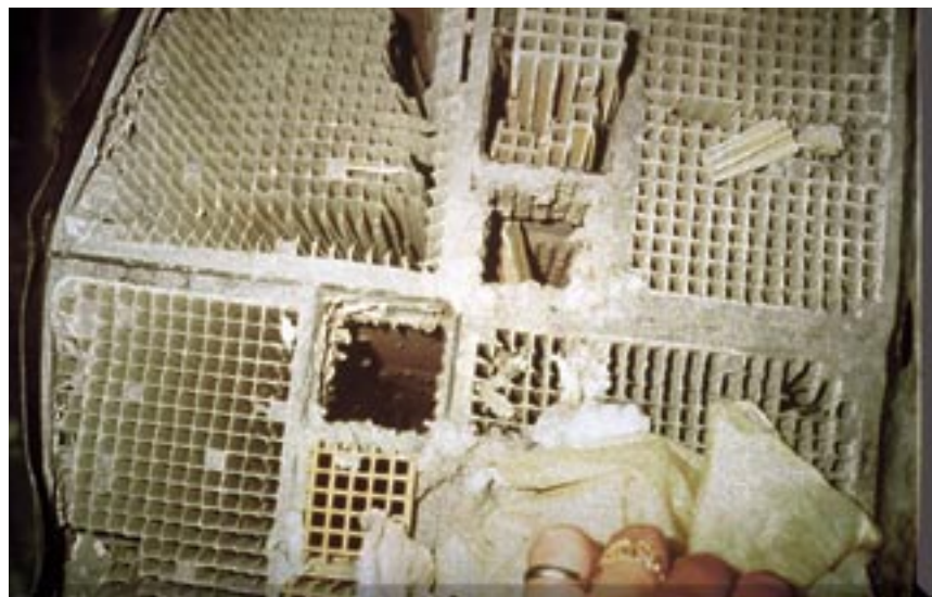
Damage caused by erosion in the catalyst bed.
