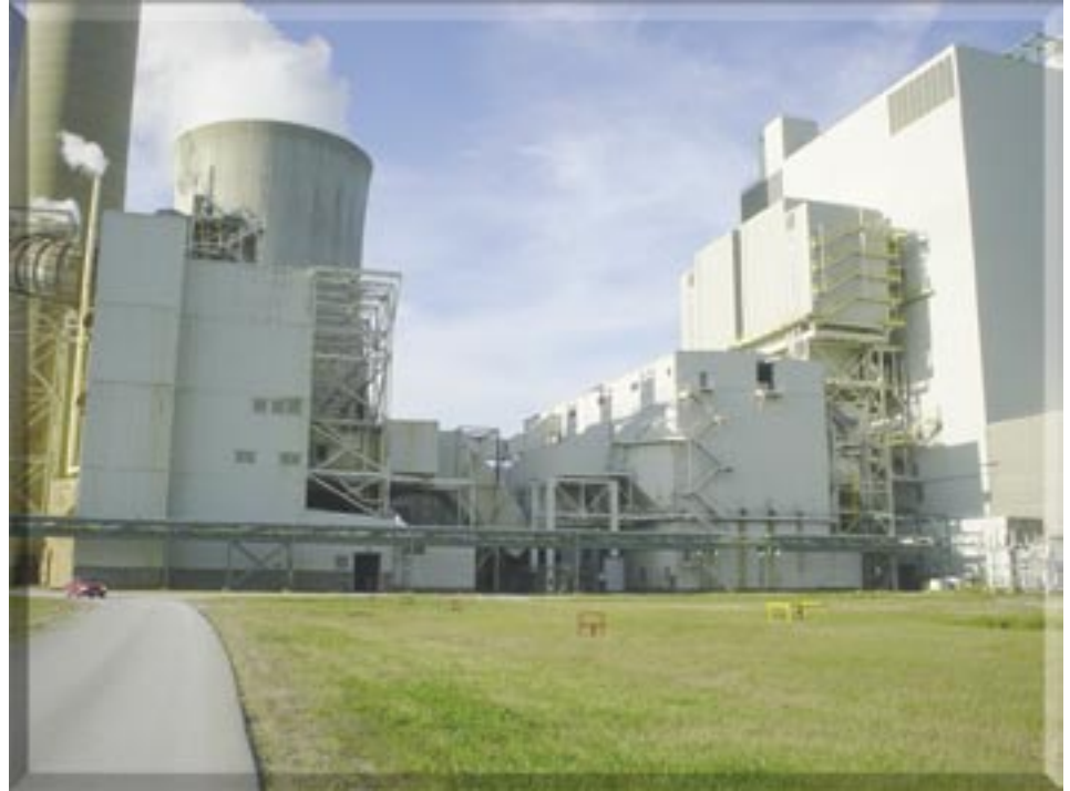
SCR unit at Trimble County 1.
