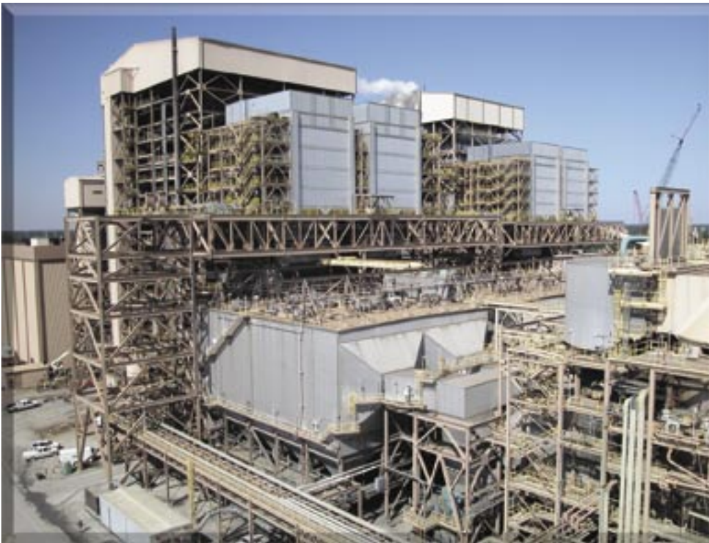
SCR units at Cross 1 and 2.
