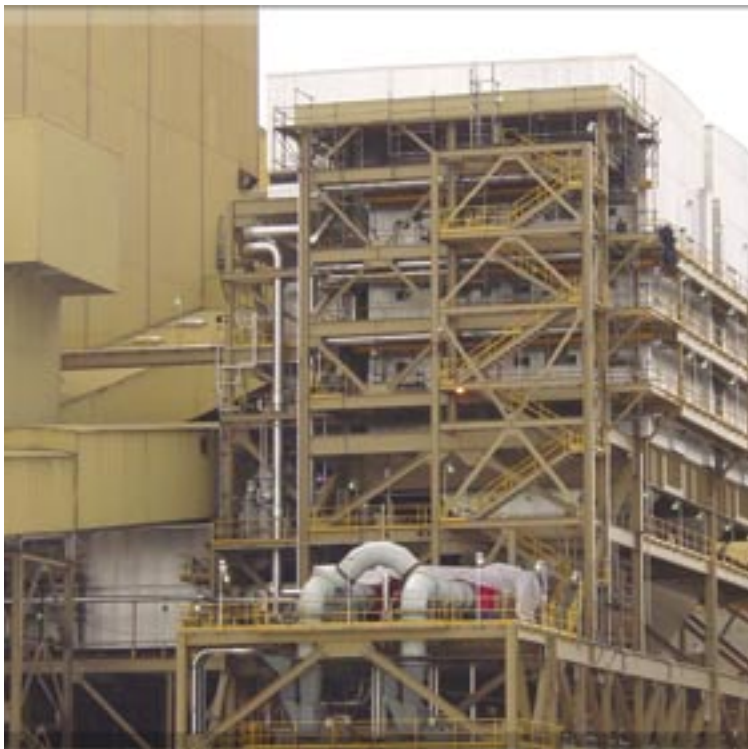
SCR unit at Ghent 1.
